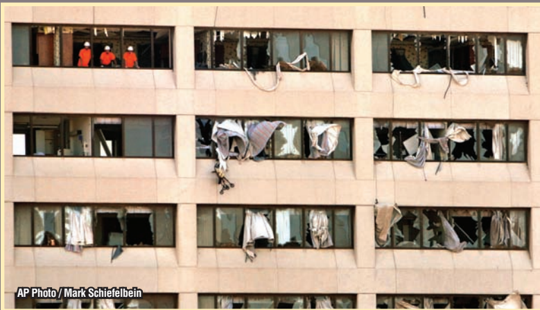
Emergency personnel look out from shattered windows in St. John's Regional Medical Center.
